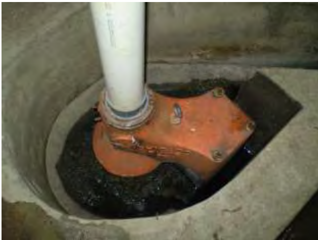
ORIGINAL CHICAGO PUMP 15C
